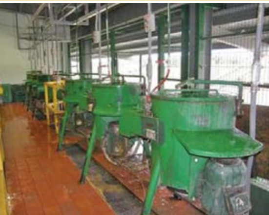
Machines used for mechanical removal of mesocarp at the new Seed Processing Unit in Coto.
